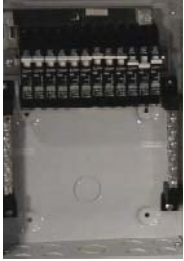
Fig. 10 Outback PSPV combiner box with twelve breakers installed.
