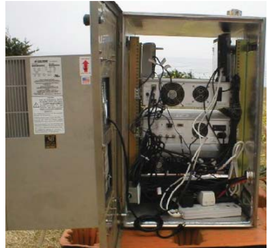
Figure 1. Interior of empty outdoor electronics enclosure without air-conditioner attached.
