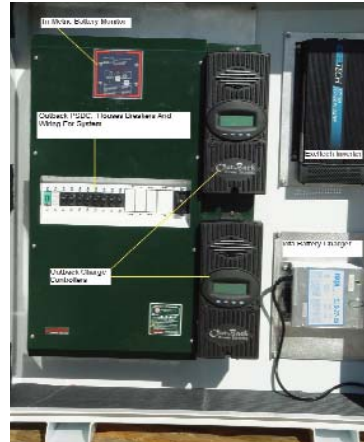
Fig. 22 Inside Enclosure Detailing Various Components
