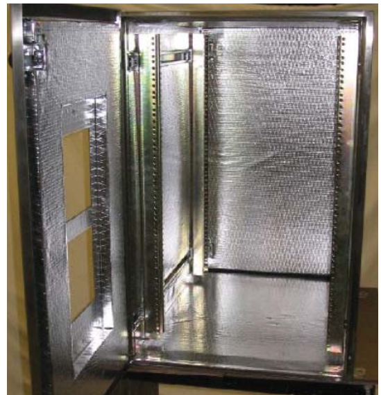
Figure 2. View of outdoor electronics enclosure with both doors open. Air conditioner is attached and all HFR electronics are mounted within the enclosure.
